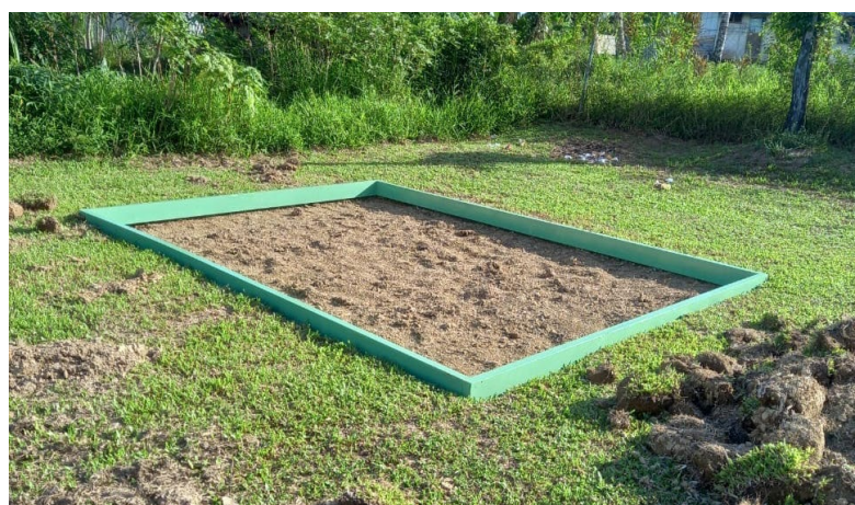
Image 5: Sandpit constructed by KTF with community help to support early childhood education.
